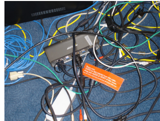
Figure 1. Wiring near the podium. Which cable should visitors use for their laptop?
